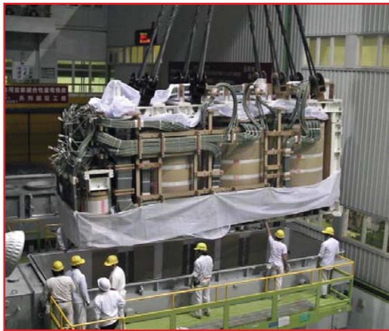
A new transformer, shown being prepared for testing, will be installed at SMECO's Hewitt Road switching station.
